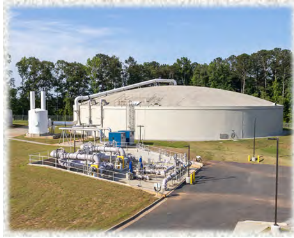
Water Treatment Facility
